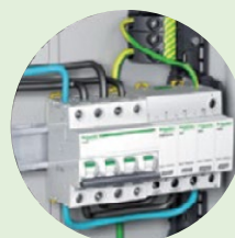
External back-up protection
