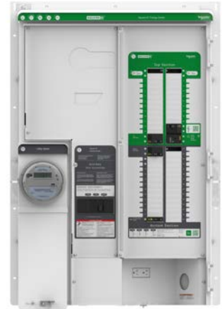
Energy Center with Cover Removed
