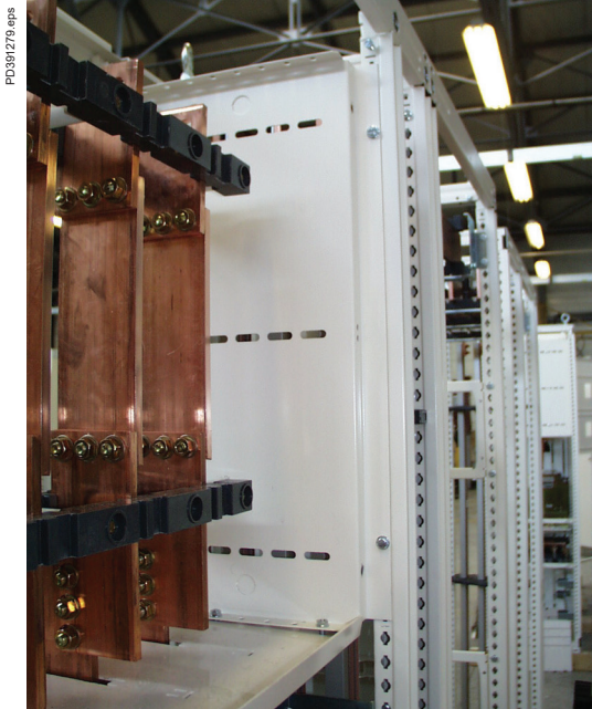
Dismountable vertical busbars.
