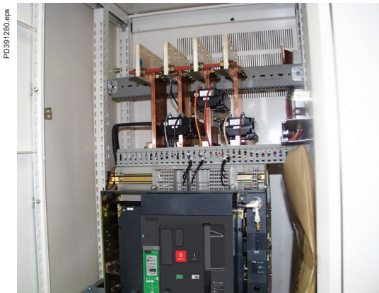
CT on vertical busbars.
