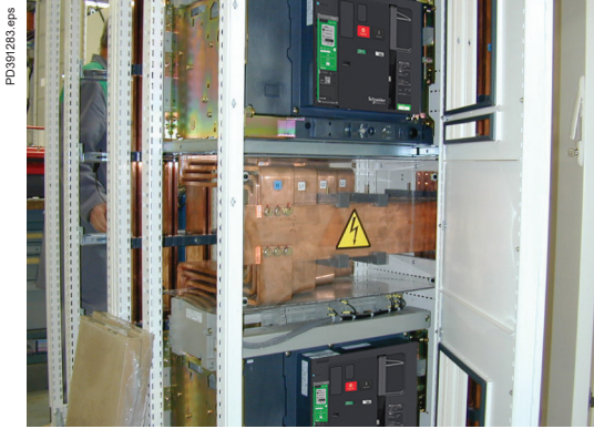
Source changeover system in the same cubicle.
